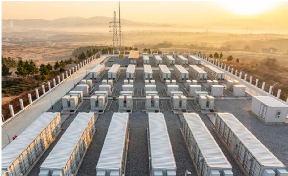
Power play Battery storage is in demand
